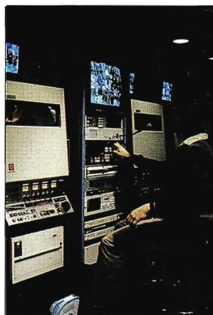
In a room adjoining Production Control, a battery of TH-200 one-inch VTRs record camera action.
