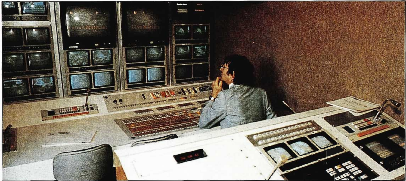
Production control in the QVLV truck features a Grass Valley 300-3A video switcher with five isolated banks and a Chyron IV graphics system.
