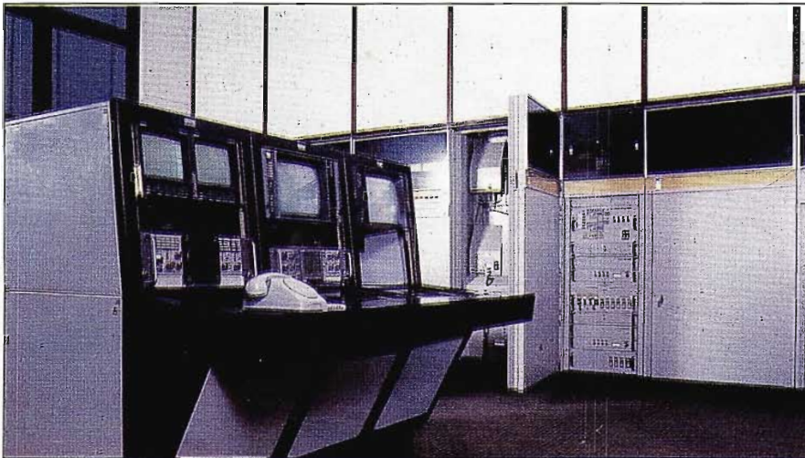
Controls for TTG-30/30L parallel transmitters are console-mounted.
